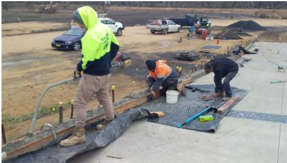
Lachlan Hall Construction Staff pouring the final kerb on truck wash down ramp
