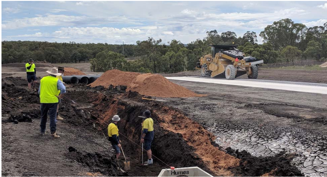
Stabilisation of all earthworks and pavement courses is being undertaken in house using Council's recently delivered CAT RM300 Pulvimixer. This pulvimixer will provide significant savings to the HPV Route construction and future Council roadworks.
