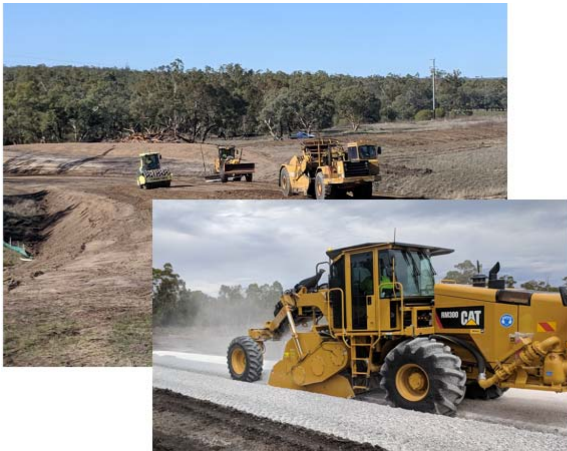
Earthworks for the entire truck wash site have been completed and stabilised, with stormwater detention works now underway. In early November Council
